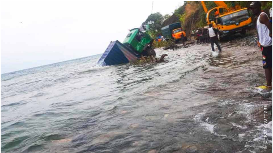
Lwanga, between Uvira and Makobola (Fizi): After heavy rains, Lake Tanganyika burst its banks and cut the road.
